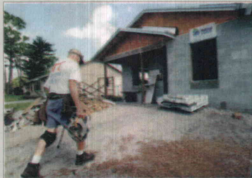
WORK GOES ON: Joe Alter, 84, of Delray Beach, heads back to work inside a Habitat home under construction west of Boynton Beach. The nonprofit agency wants to combine its administrative office and the Re-Store at the Delray Beach warehouse. Staff photo/Mark Randall
